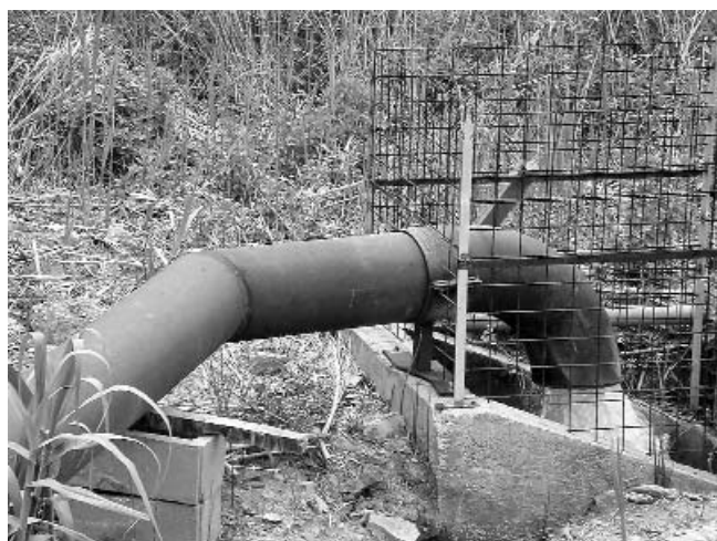
Figure 23. Water pumping system at the Gavorrano underground mine (at present, about 80 L/s)
