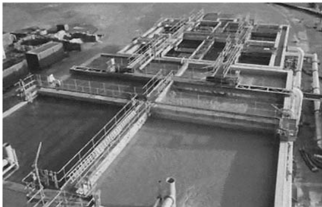
Figure 31. Wheal Jane HDS plant showing the reactors and lamella clarifiers
