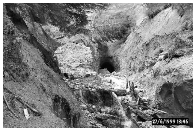
Figure 15. Same water outlet after water outburst
