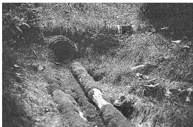
Figure 14. Water outlet before water outburst in 1998
